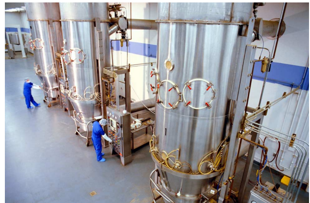
Storage Tanks (Outstations)
